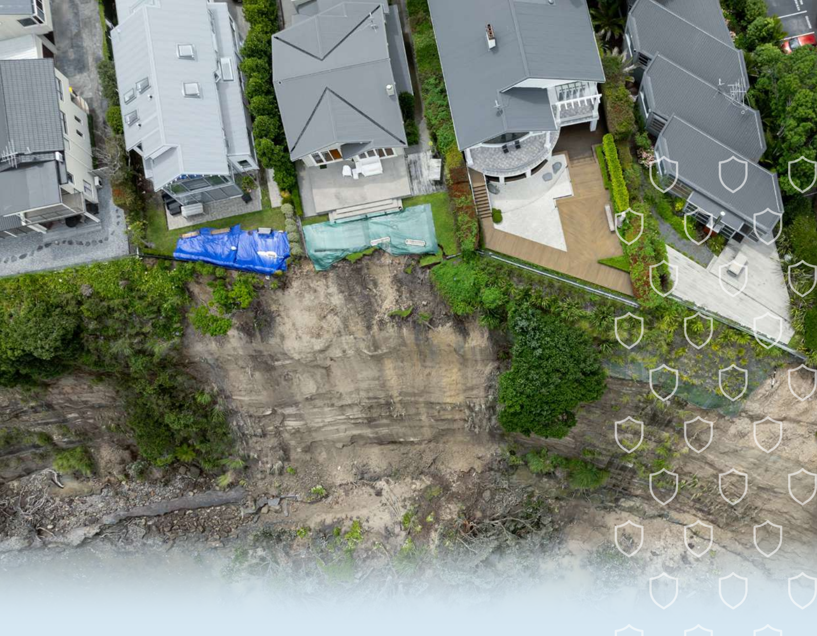
Erosion flood damage at Stanley Point, Auckland after the Auckland Anniversary floods, 2023
