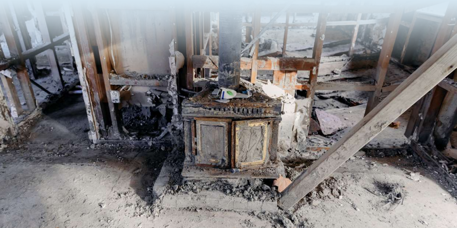
Interior of a house destroyed by flooding from Cyclone Gabrielle, Eskdale, Napier, Hawkes Bay
